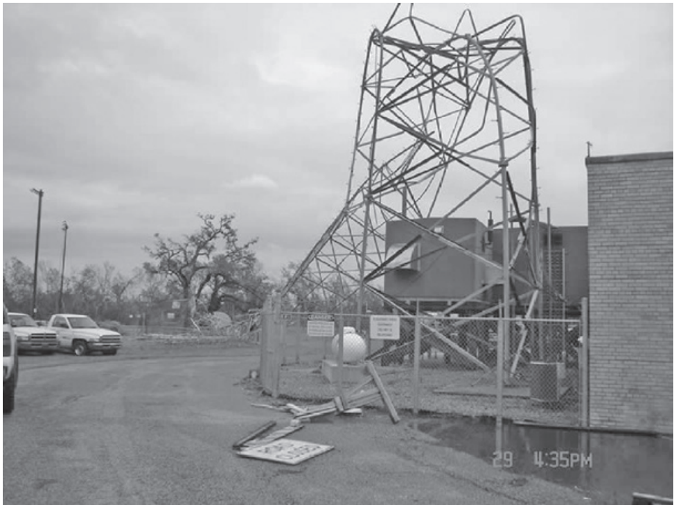
Figure 16-8: Plaquemines Parish (Louisiana) Radio Tower – August 29, 2005
